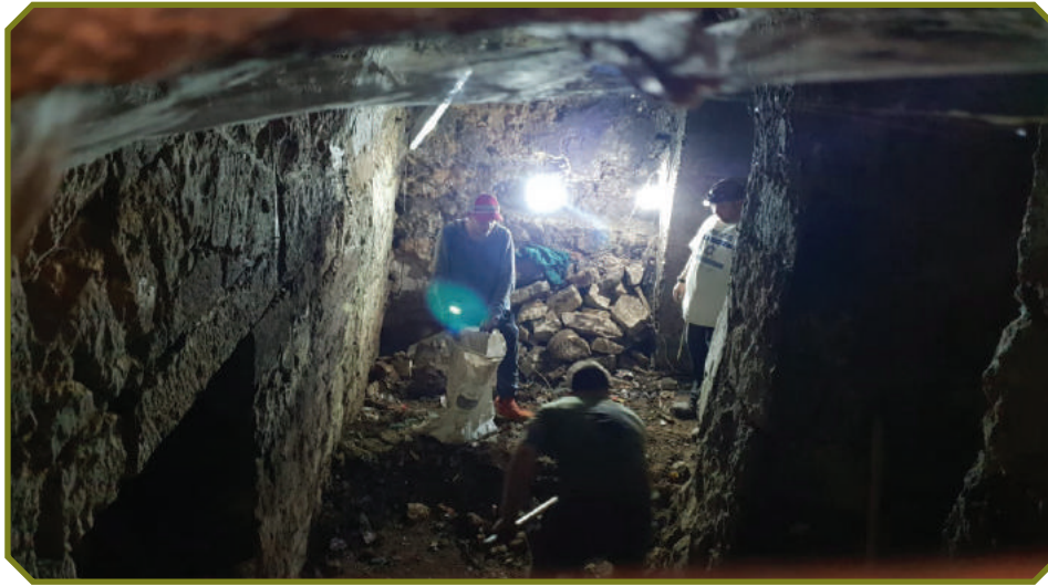
EXCAVATIONS CARRIED OUT BY THE SETTLERS INSIDE A BASEMENT UNDER THE HOUSE OF THE ZA'TARI FAMILY
