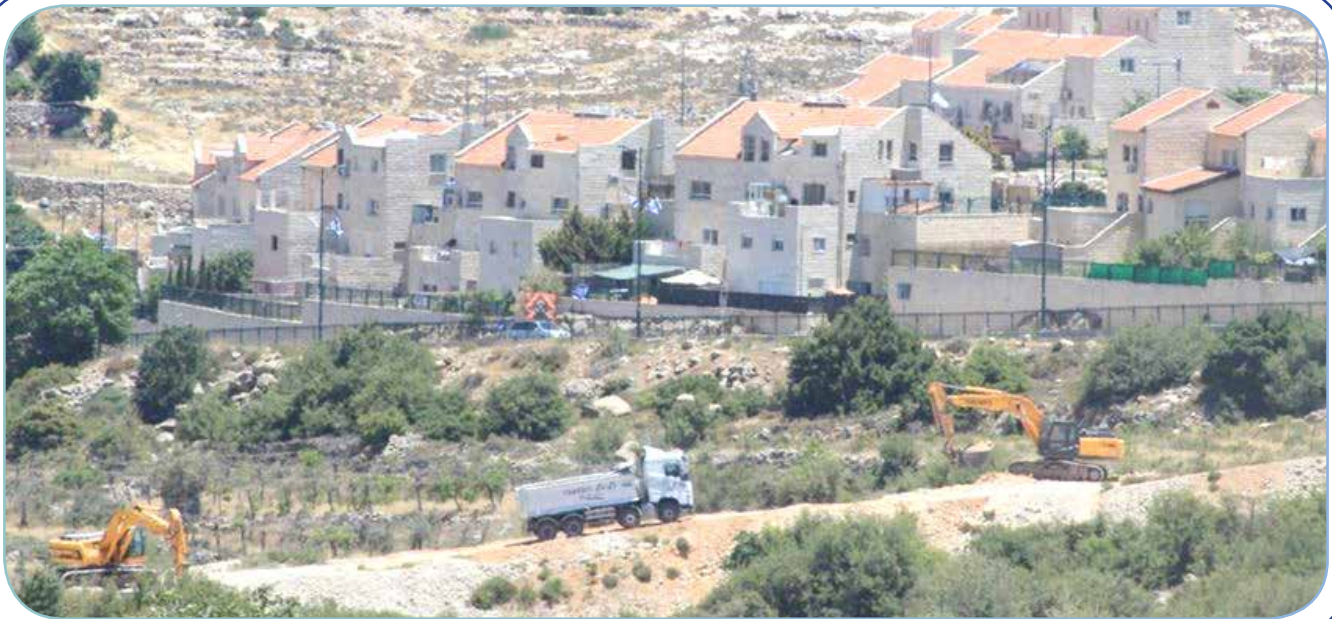
Imageε: An Israeli bulldozer removing construction scrapings upon the issuance of the decision
