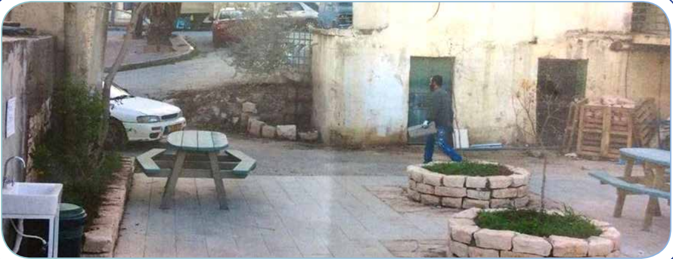
Image1: The renovation work by settlers at the gas station in preparation of taking it over.
